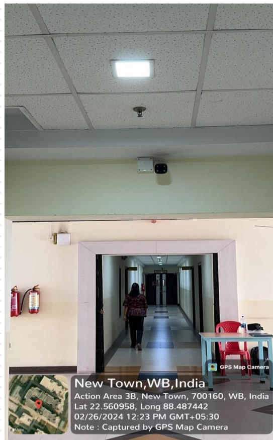
CCTV camera in the Corridor
